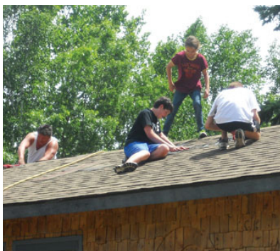
Robert Durant, tribal council member of the White Earth Tribe, together with his daughter and two high school members from St. Luke's Church of Darien, Conn., finish the roof on Earl's home.
